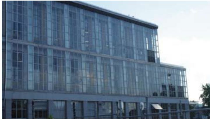
Figure 43 Exterior glass curtain wall at the National Printing Bureau (c1950). The curtain wall is part of a double-wall assembly intended to help control interior conditions within the printing and production areas. Gatineau, Quebec. Source: MTBA Associates Inc.
