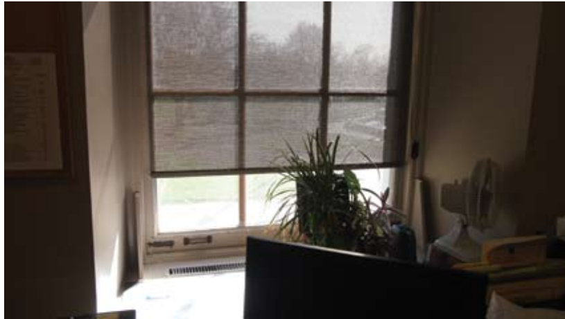
Figure 17 Localized control of sun-shading, heating, window operation, and air movement, Frontenac County Courthouse, Kingston, Ontario.
