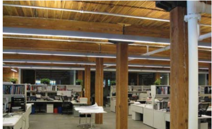
Figure 78 The wood structure and flooring system were retained in adaptive reuse. Former McGregor Sock Factory (Stantec Offices) Toronto, ON. Source: MTBA Associates Inc.
