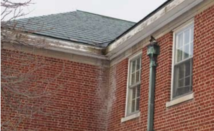
Figure 42 Exterior walls, especially at interior corners, have been exposed to significantly increased amounts of water from the roof valley due to the loss of eaves troughing. As a result, the mortar is failing and the brick cladding is spalling. In addition, opportunities to collect rainwater for grounds maintenance are lost. Sagonaska School, Sir James Whitney School, Belleville, ON.
