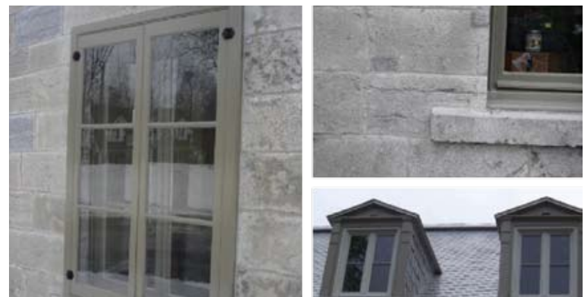
From top left: New storm window based on original design installed to improve existing window performance. Repointed and repaired masonry. Rehabilitated dormers with new windows.
