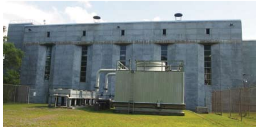
Figure 35 North elevation showing later chiller addition placed without regard for the strong axuality and Beaux-Arts planning, which is a character-defining element of the FHBRO “Classified” property. National Printing Bureau Central Heating Plant, Gatineau, QC. Source: MTBA Associates Inc.
