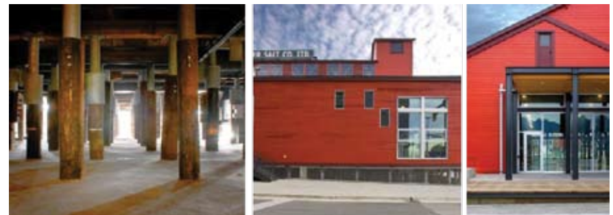
Left to right: Building raised 1 metre with 300 steel pile extensions; view of piles and new and old windows; restored façade and new covered area
