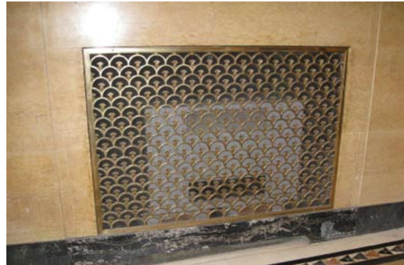
Figure 67 Ornamental bronze radiator covers conceal mechanical equipment and offer opportunities for equipment upgrades without altering visual appearance. Canada Permanent Building, Toronto, ON. Source: MTBA Associates Inc.
