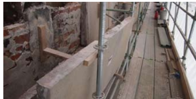
Figure 77 Limestone cladding, masonry back-up, and steel structure, each impacting the other. Sir John A Macdonald Building, Ottawa, ON. Source: MTBA Associates Inc.
