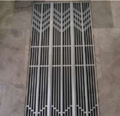
Figure 81 Architectural metal grille. College Park Building. Toronto, ON. Source: MTBA Associates Inc.
