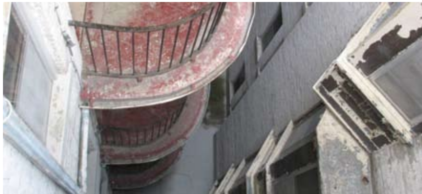
Figure 59 Light wells and light courts, such as this one at the Roslyn Courts National Historic Site, Winnipeg, MB, are an effective means to provide natural light and ventilation in a multi-storey building. The light coloured walls are highly reflective which encourages more efficient use of natural light. Source: Shelley Bruce
