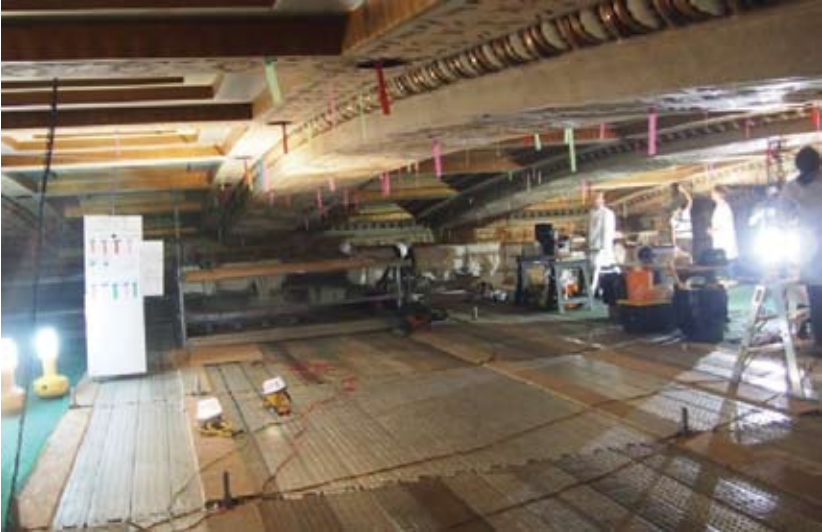
Figure 83 Conservators performing on-going rehabilitation of a plaster ceiling and plaster finishes. Sir John A Macdonald Building, Ottawa, ON. Source: MTBA Associates Inc.
