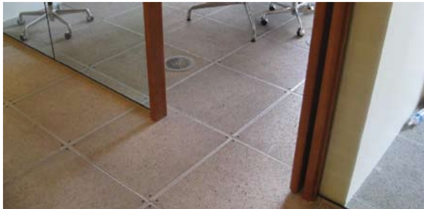
Figure 63 Raised floor system installed in historic building. Former McGregor Sock Factory (now Stantec Offices), Toronto, Ontario. Source: MTBA Associates Inc.
