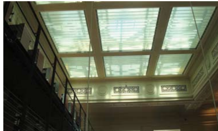
Figure 57 Large central skylight in a banking hall. The skylight provides natural light to the hall, which is located mid-block with limited access to street front windows. The skylight was uncovered during rehabilitation of the former Bank of Nova Scotia, Ottawa, Ontario. Source: MTBA Associates Inc.
