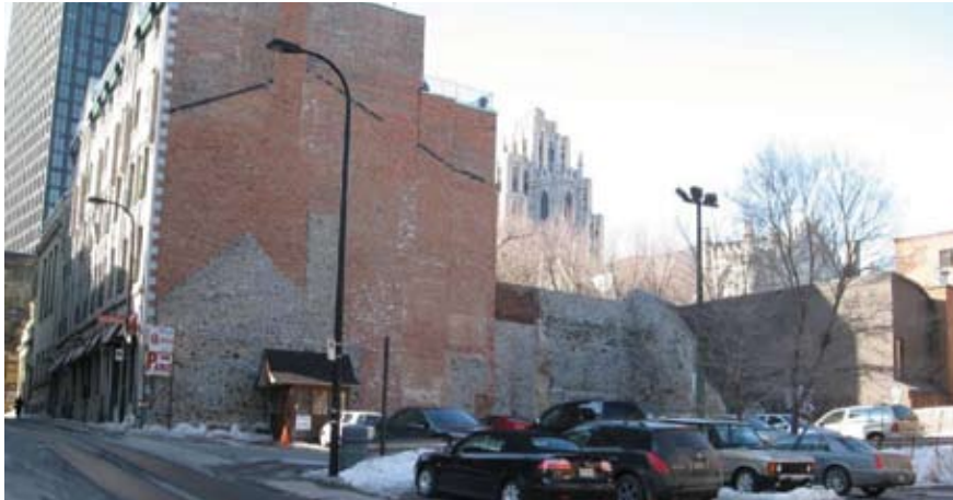
Figure 32 An example of urban scarring where evidence of building evolution can be seen on an adjacent property. Changes to adjacent buildings can expose walls never intended to be exposed. Montreal, QC. Source: MTBA Associates Inc.
