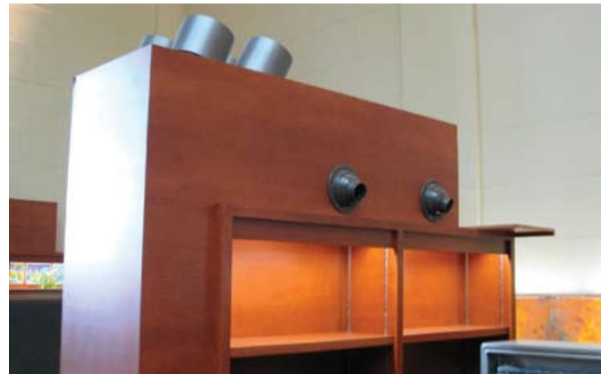
Figure 87 Directional localized Punkah grilles integrated into modern furniture insertions within a voluminous former banking hall. Library of Parliament Annex (Former Bank of Nova Scotia Rehabilitation), Ottawa, ON. Source: MTBA Associates Inc.
