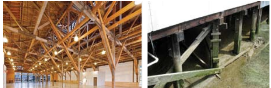
Figure 38 (left) Rehabilitated long span wood trusses. The timber truss system was repaired by replacing defective or missing members and installing steel plates at connection points. Thus, this significant character-defining element was retained along with the old growth timber. As part of the rehabilitation process the building foundation was modified altering its relation to the ground plane. The new foundation system is clearly legible on the building exterior. For more information refer to the case study at the end of this document. Salt Building, Vancouver, BC. Source: Acton Ostry
