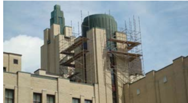
Figure 76 On-going rehabilitation on the exterior masonry wall envelope. Université de Montréal. Montreal, QC. Source: MTBA Associates Inc.
