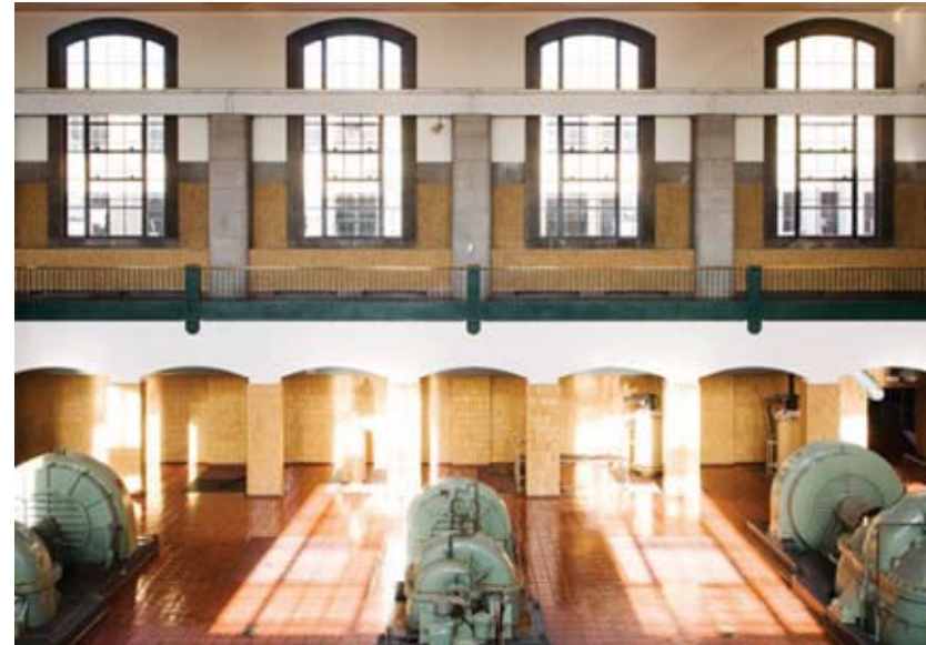
Figure 66 Active pumping equipment integrated into the water filtration process, while also being celebrated as significant objects within the light-filled room. . RC Harris Water Filtration Plant. Toronto, ON. Source: Torontist
