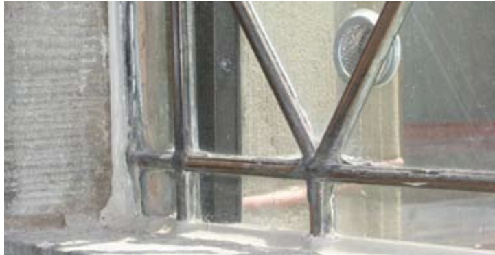
Figure 51 Window detail with puttied muntins, perimeter sealant and vented exterior storm window. Canadian Museum of Nature, Victoria Memorial Museum Building, Ottawa, ON. Source: Shelley Bruce
