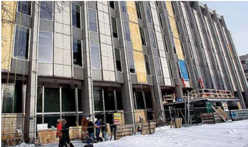
Figure 46 Rehabilitation of exterior envelope including full removal of all granite cladding panels to install new exterior insulation proud of the structural steel. The resulting 125mm shift is accommodated by a stainless steel channel added on the side elevations. Workers Compensation Board, Winnipeg, MB. Source: 1x1 Architecture
