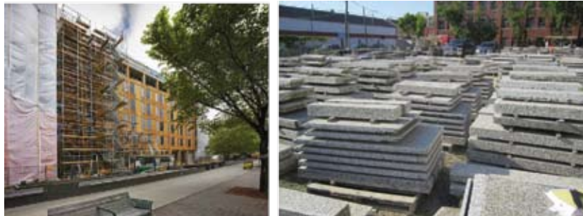
Left to Right: Temporary plywood panels provide a barrier to the elements during construction, hoarding provided containment during asbestos removal. A total of 4044 original granite panels were cleaned, catalogued and stored off site.
