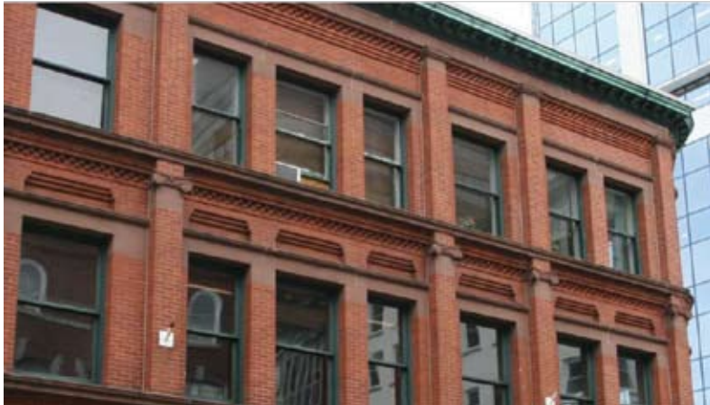
Figure 85 Operable upper storey windows in a mixed use heritage building. Halifax, NS. Source: Shelley Bruce
