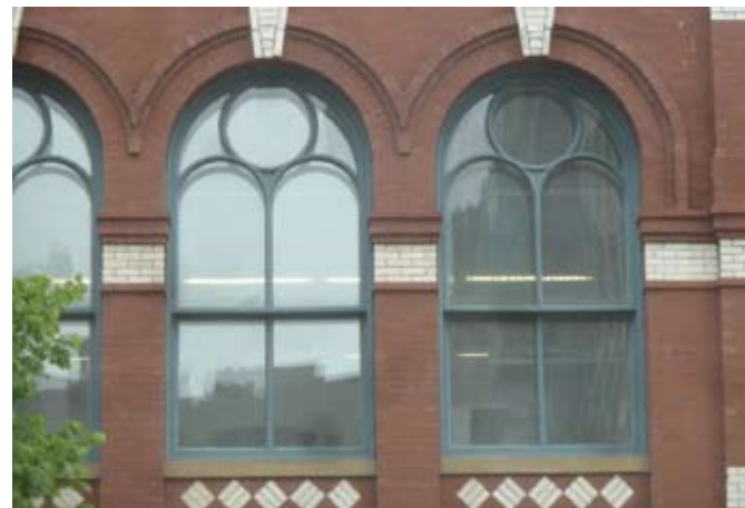
King St. window detail. Energy panels were installed on the interior to improve thermal performance while also retaining these character-defining elements . Source: Jim Bezanon
