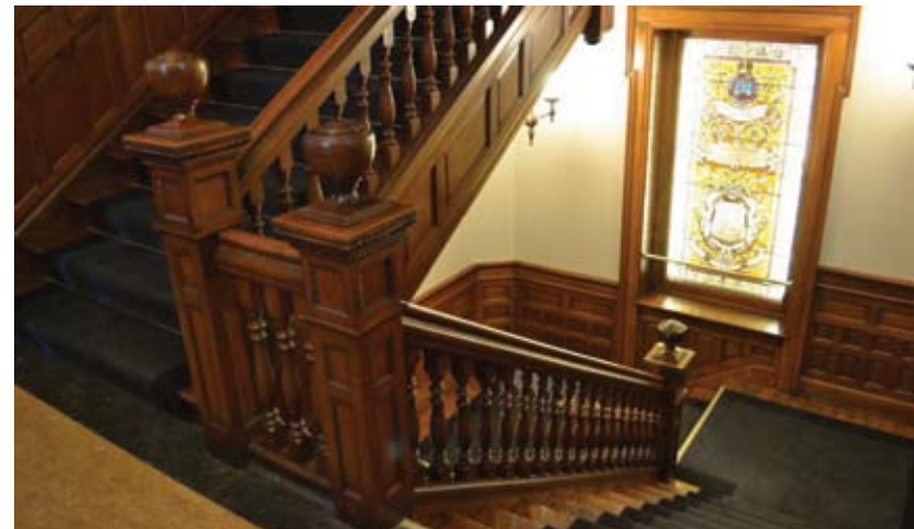
Figure 72 Architectural woodwork retained as part of a rehabilitation and addition. Elgin County Courthouse, St. Thomas, ON. Source: FGMDA
