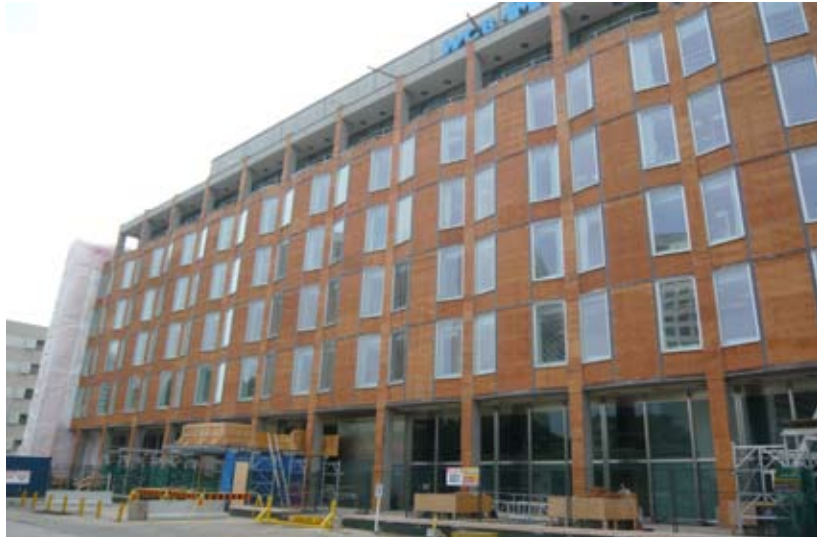
Figure 24 Full exterior envelope rehabilitated. Image shows rehabilitation progressing with granite panels temporarily removed to allow for the installation of new insulation and other envelope upgrades. For more information on the rehabilitation, refer to the Case Study found in the Case Study Appendix of this document. 333 Broadway, Winnipeg, MB. Source: Winnipeg Architecture Foundation.
