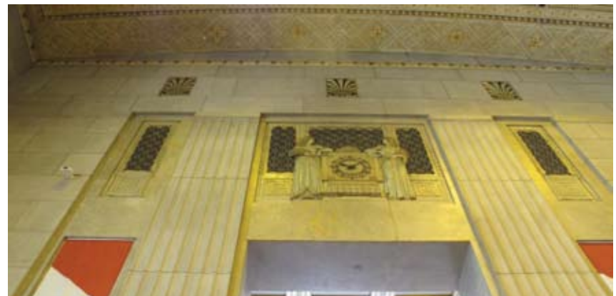
Figure 62 Ornamental plaster ventilation grilles in the main banking hall were formerly connected to large fan units above and behind. Grilles were rehabilitated and integrated into the new mechanical system as exhaust grilles. Sir John A Macdonald Building, Ottawa, ON. Source: MTBA Associates Inc.
