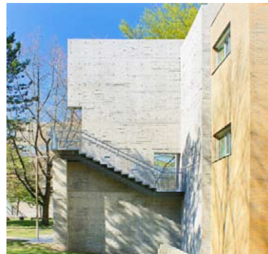
Figure 27 New seismic buttress connected to the existing building. Friedman Building, University of British Columbia. Source: Acton Ostry
