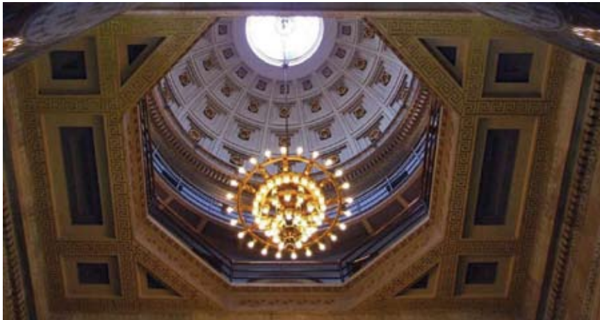
Figure 37 Interior view of double-shelled dome, a character-defining element, allowing air stratification and access to natural light at the Bank of Montreal head office, Montreal, QC. Source: MTBA Associates Inc.
