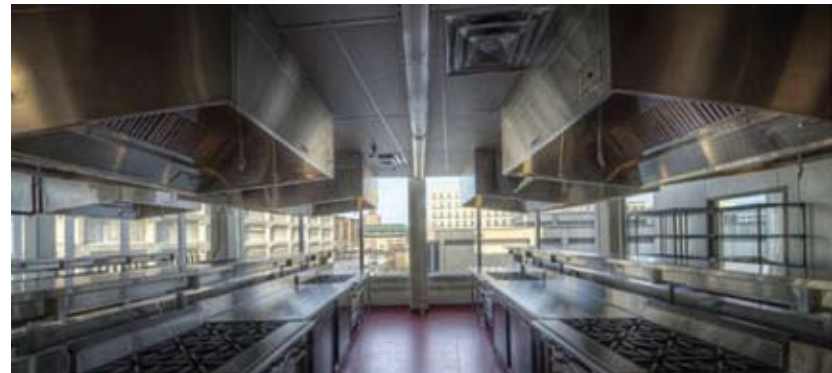
Figure 65 New kitchen exhaust equipment is integrated in the building's overall HVAC system to capture waste heat generated from cooking activities. Paterson GlobalFoods Institute (Former Union Bank Tower), Winnipeg, MB. Source: Prairie Architects
