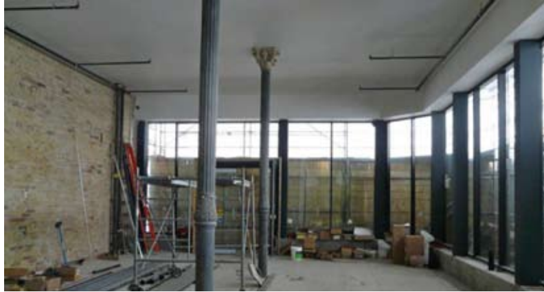
Figure 70 Ground floor commercial space under rehabilitation . Ceiling height pulled back to original to expose decorative column capitals and accommodate taller storefront windows, allowing natural light to penetrate deeper into the space. Dineen Building. Toronto, ON. Source: Urban Toronto
