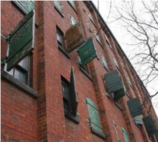
Figure 52 Industrial buildings like this one in Toronto have shutters to protect the windows and to retain heat. Toronto, ON. Source: Shelley Bruce
